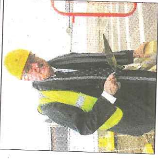
Housing boss, Cllr Howard Doe, lays the first brick at St Mary's Island development
